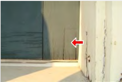
K. Picture 11 Weather Damage at Door
