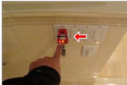
E. Picture 8 Defective GFCI
