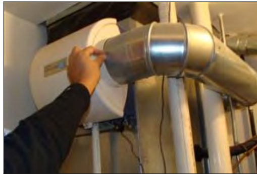
G. Picture 11 Missing Damper
