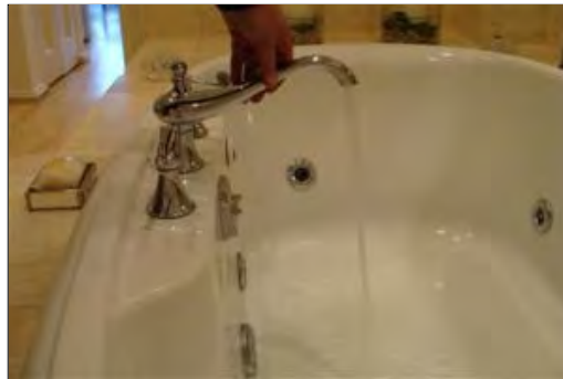
F. Picture 11 Loose Spout
