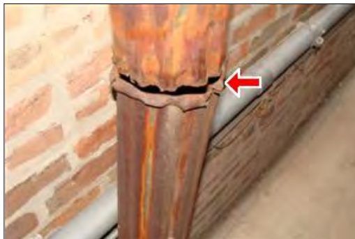
C. Picture 8 Open Downspout Joint
