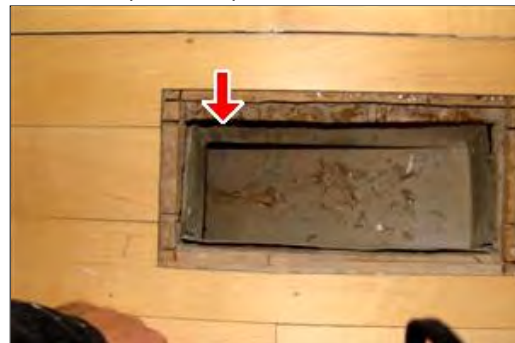
G. Picture 7 Gap at Register Boot
