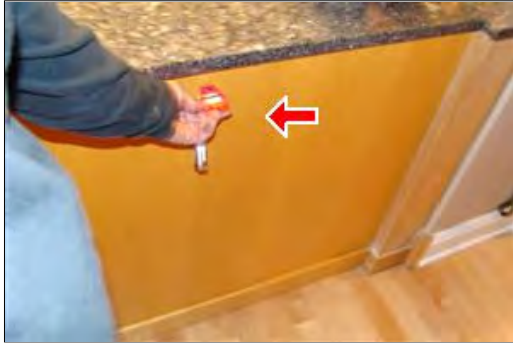
E. Picture 5 Missing Receptacle
