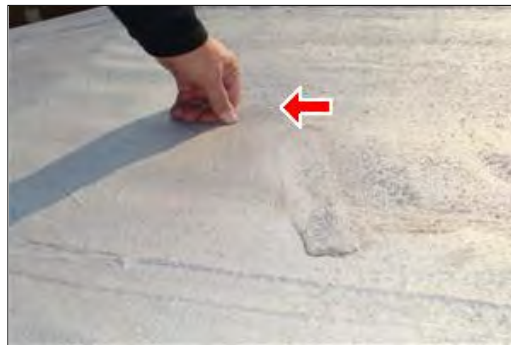
C. Picture 1 Spongy Roof Deck
