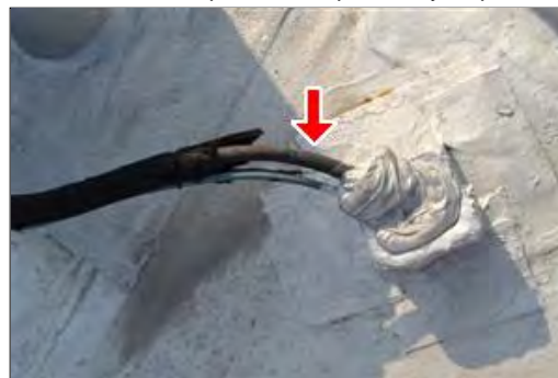
G. Picture 1 Missing Insulation
