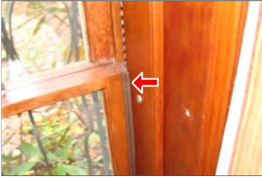
K. Picture 8 Loose Weatherstripping
