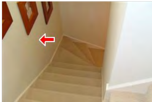
J. Picture 8 Missing Railing
