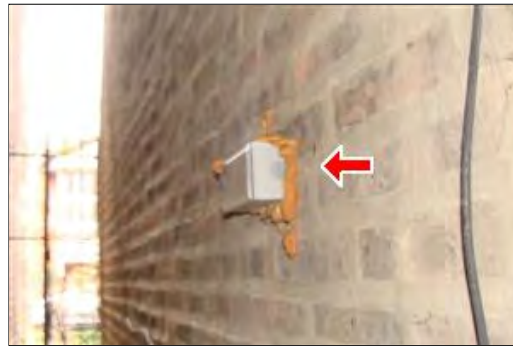
A. Picture 25 West Wall Junction Box
