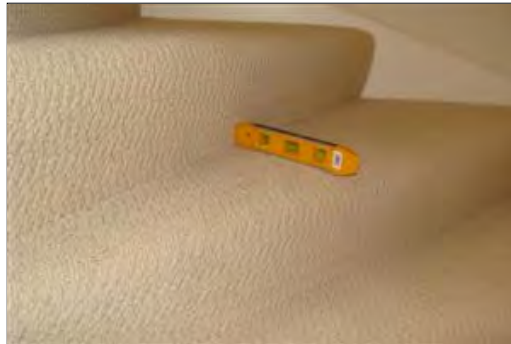
J. Picture 3 Excess Tread Slope
