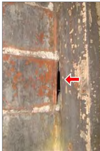
A. Picture 17 Missing Caulk
