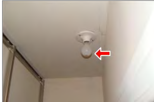
E. Picture 2 Closet Light Fixture
