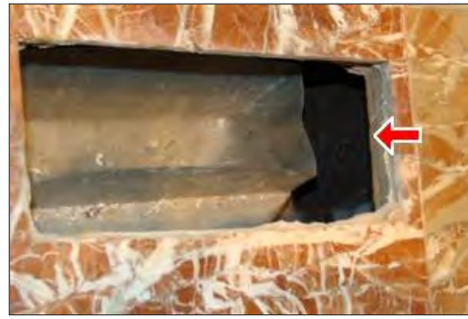
G. Picture 9 Sunken Duct and Boot
