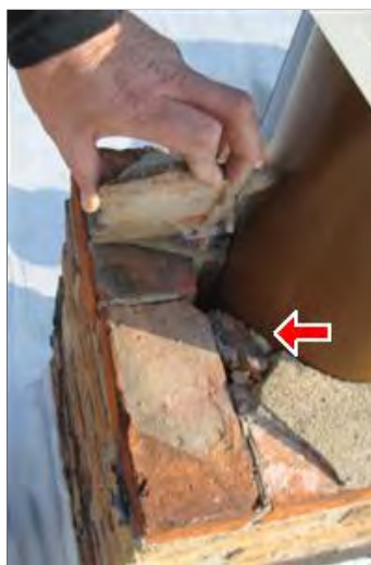
A. Picture 8 Chimney Deterioration
