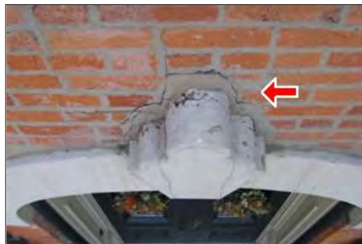
A. Picture 22 Mortar Cracking
