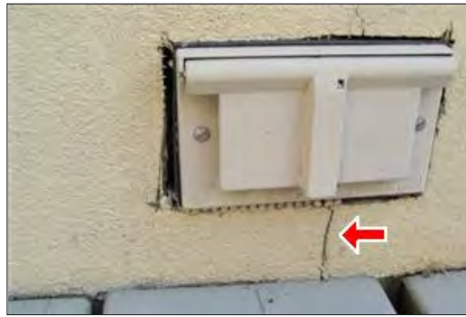
A. Picture 19 Stucco Cracking
