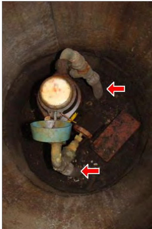
F. Picture 10 Lead Piping in Vault
