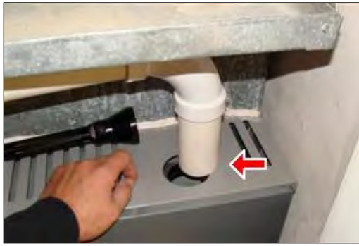
G. Picture 2 Top Floor HVAC Unit
