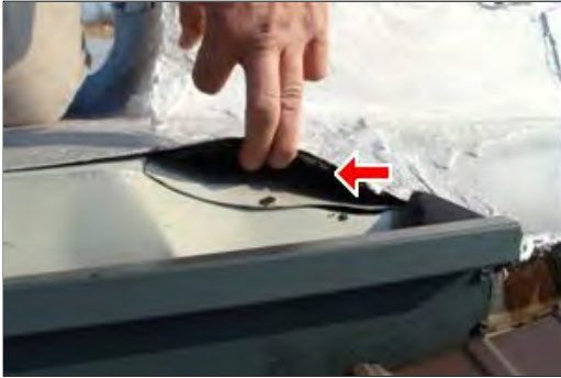
C. Picture 5 Unsealed Roof Membrane
