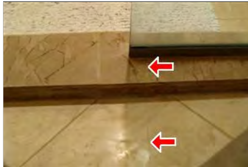
J. Picture 7 Tile Cracking and High Moisture
