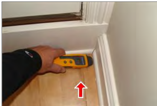
A. Picture 13 Elevated Moisture at Wood Floor
