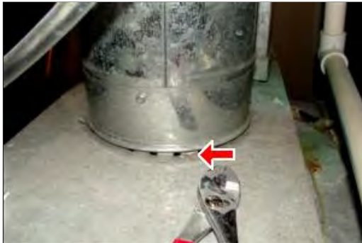
G. Picture 3 HVAC Duct Gaps
