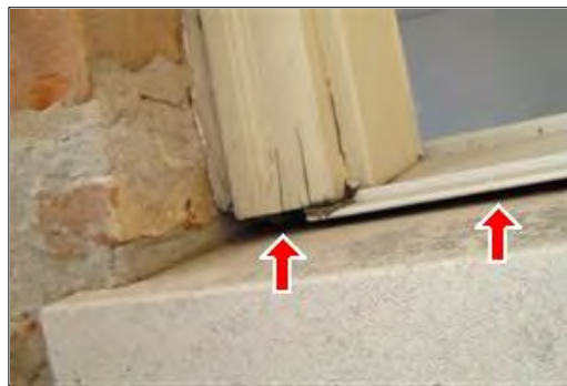
K. Picture 13 Missing Sealant at Balcony Door
