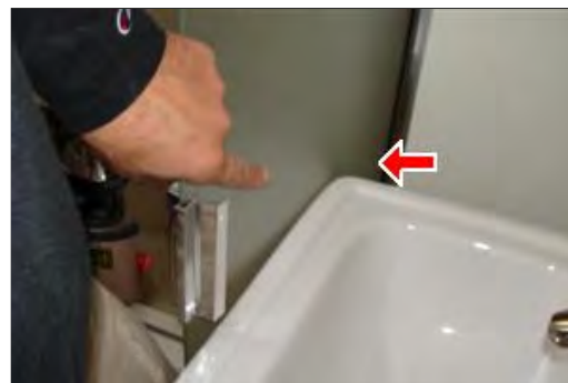
J. Picture 1 Breakage Hazard
