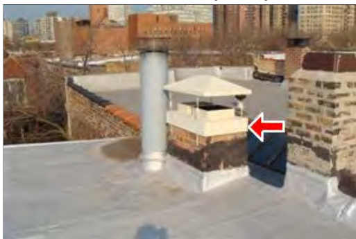
H. Picture 1 Two Flue Chimney
