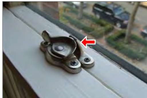
K. Picture 7 Broken Window Latch
