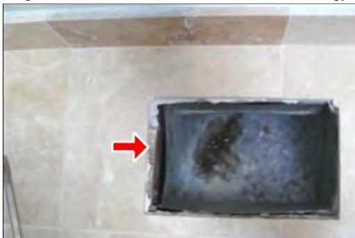
G. Picture 6 Gap at Register Boot
