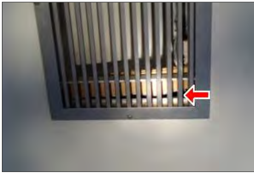
G. Picture 8 Large Gap at Return Register
