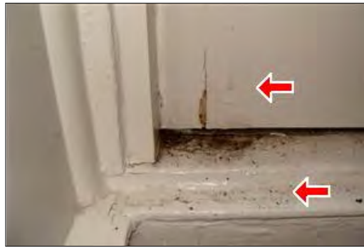
K. Picture 10 Painted-over Damage at 1st Floor North Wall Window
