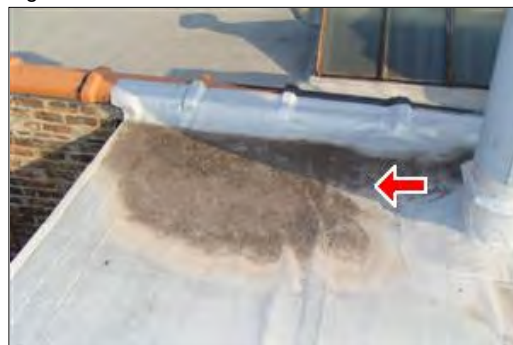
C. Picture 3 Ponding Evidence
