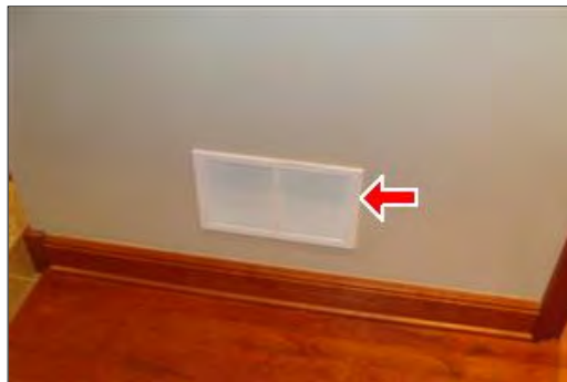
G. Picture 13 "Panned" HVAC Air Return
