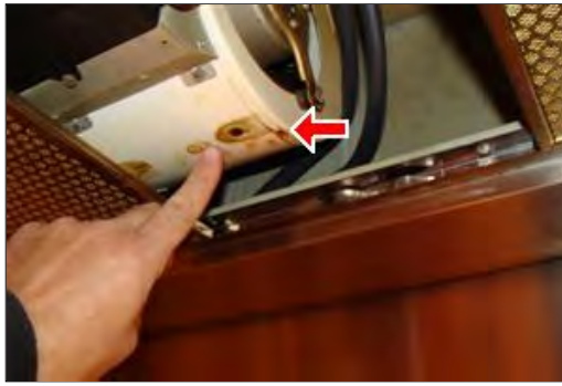
L. Picture 3 Grease at Exhaust Fan
