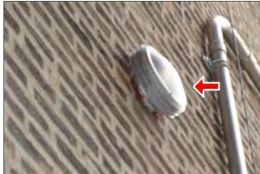
F. Picture 8 Kitchen Range Hood Vent Termination
