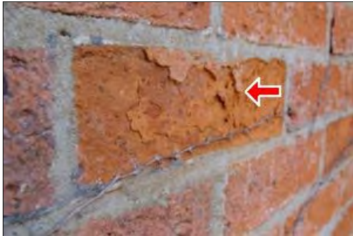
A. Picture 20 Flaking Brick
