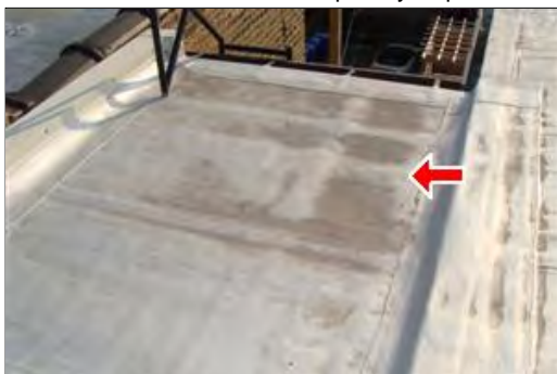
C. Picture 2 Ponding Evidence
