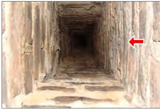
H. Picture 3 North Flue
