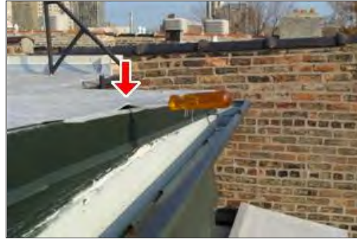
C. Picture 6 Gap at Roof Edge
