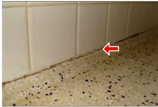
J. Picture 2 Degraded Caulk
