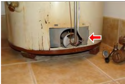
F. Picture 3 Missing Cover
