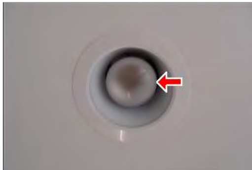
I. Picture 3 Can Lighting at Top Floor
