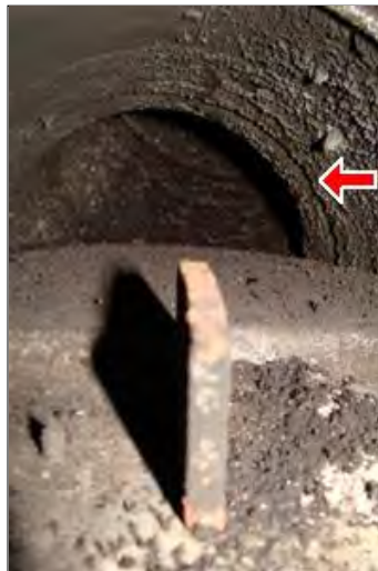
H. Picture 5 Accretions Inside Living Room Fireplace Flue
