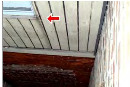
K. Picture 5 Plywood Siding at East Elevation Light Well
